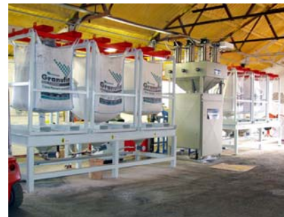
Colourtone Processing Plant
